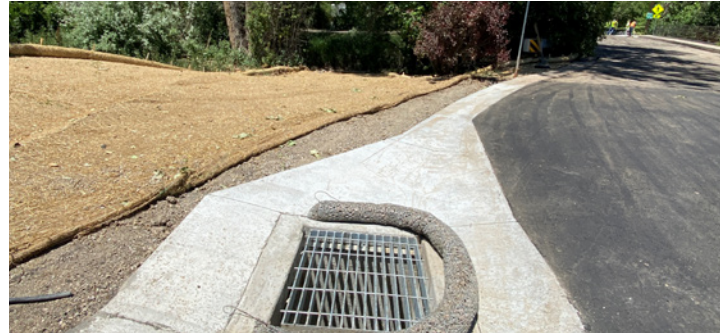
Stormwater Infrastructure, Littleton
